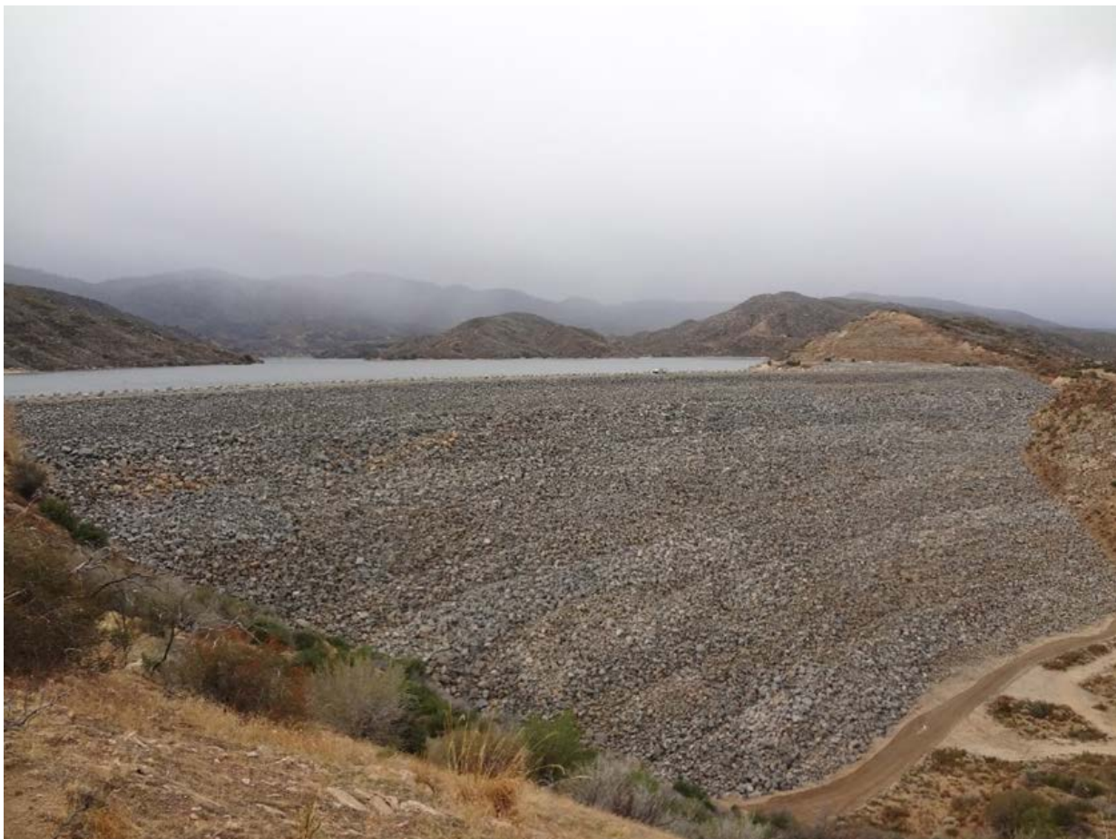
Figure 3.1-1. Downstream Face of Cedar Springs Dam and Silverwood Lake from the Right Abutment
